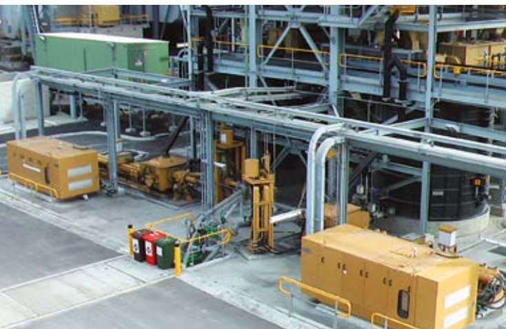
KOS pump system for fly and ground ash (Kogan Creek, Australia)
