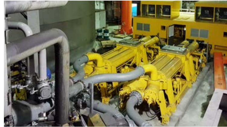
2 x HSP conveying iron ore concentrate across a distance of 26.5 km, Stary Oskol, Russia
