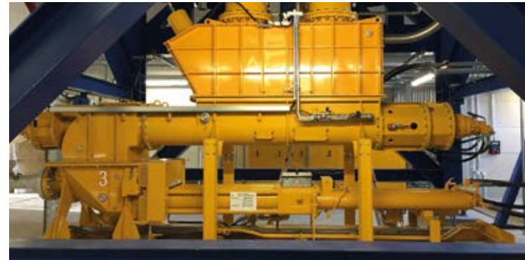
KOS with THS and JT in the Kassel power station
