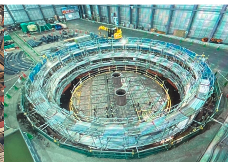
A current picture of the construction site: This is a vertical shaft of the municipal sewage system for a residential area.
